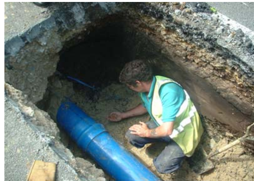
Leaking joint identified using Sahara
