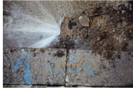
A leak on a 24" main
